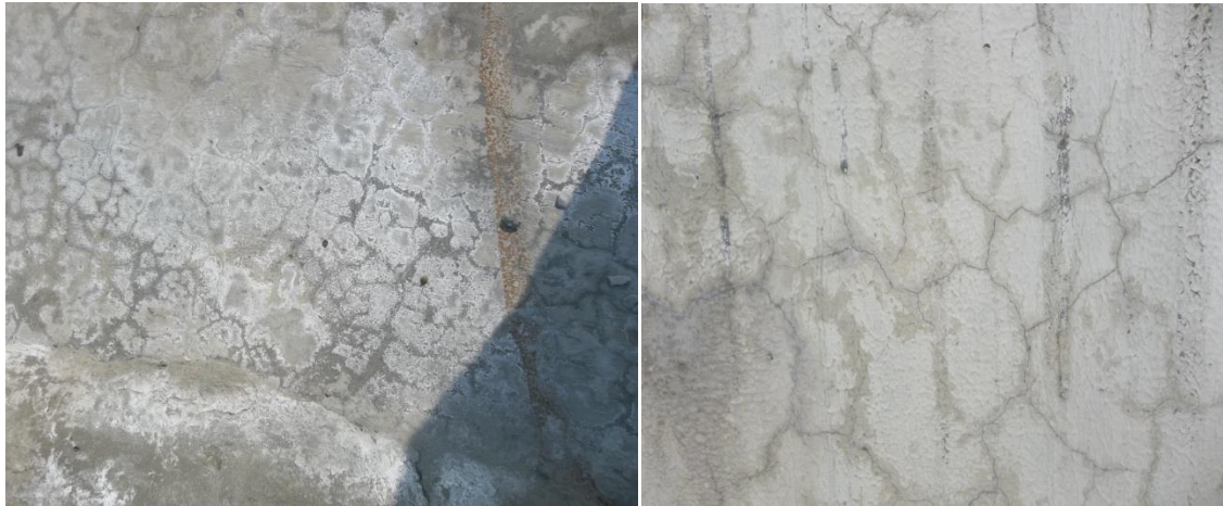
Fig. 1.1: White efflorescence on water tank slab and cracks on side wall
